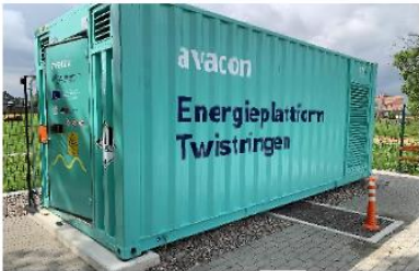
Provision flexible power and storage capacity
